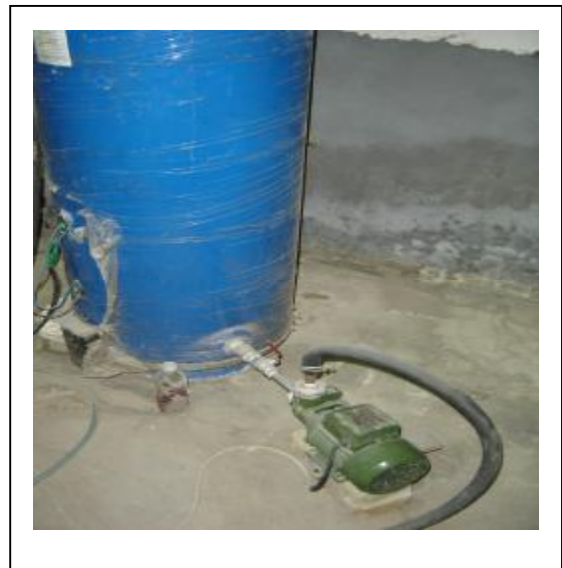
Fig. 8. Water Pump and Heater.
